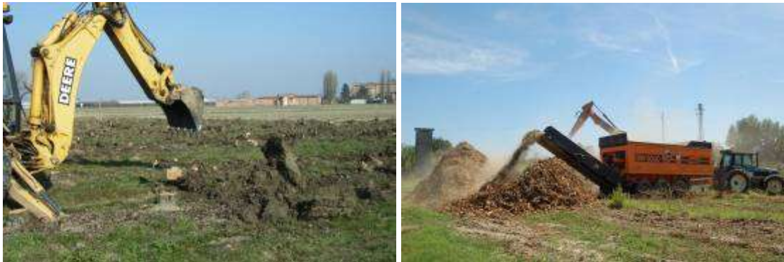
Figure 03-01 7: Common uprooting procedure by mean of excavator (left) and stump comminution by mean of grinder (right) (source: Gianni Picchi).
