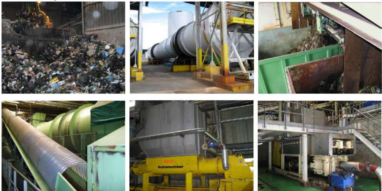
Figure 03-03 1: Dry digester material handling equipment.
