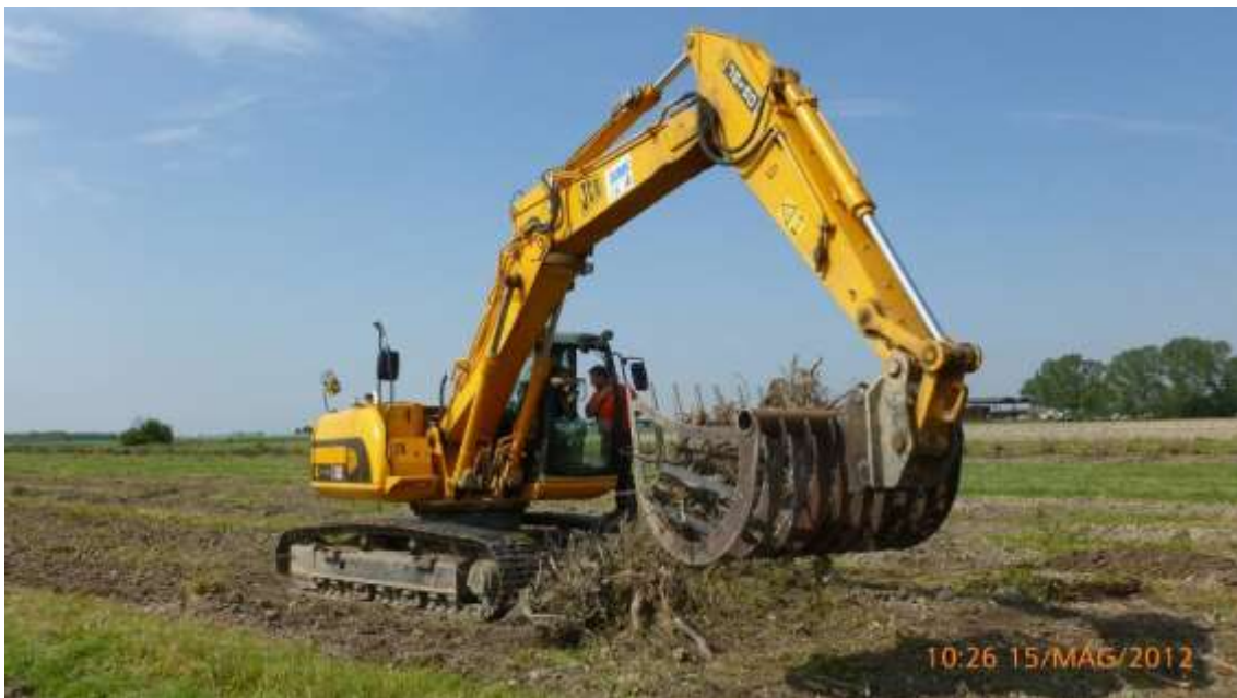
Figure 01-01 16: Stump biomass can be roughly cleaned by impurities with an appropriate handling (source: Picchi)
