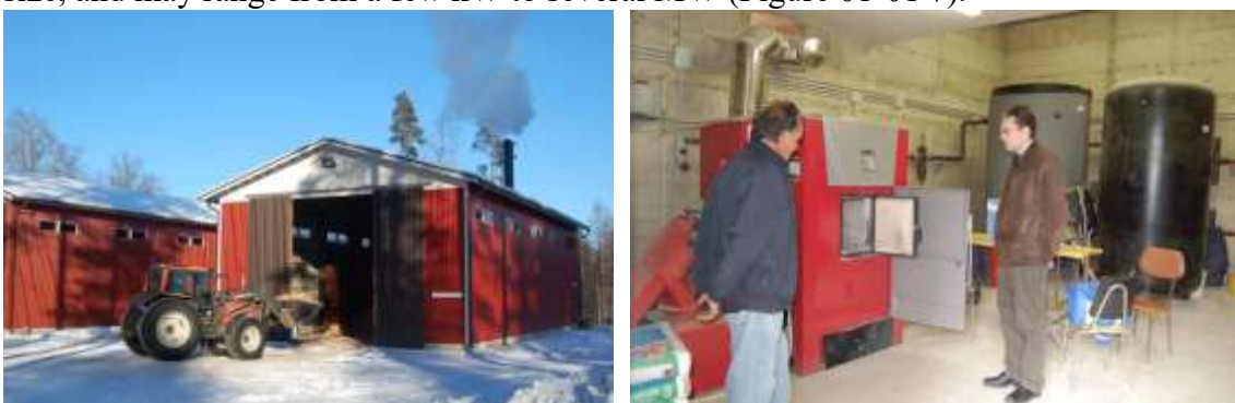
Figure 01-01 7: Two examples of wood chips appliances: a small district heating in Finland (left, note the wood chips deposit and the front loader moving the fuel) and a domestic boiler for heating a rural tourism complex in Italy (right) (source: Picchi)
