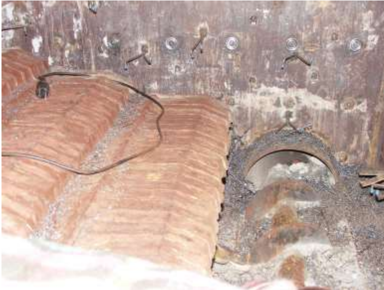
Figure 04-00 7: The lower portion of the grate in moving-grate boiler with the ash screw.
